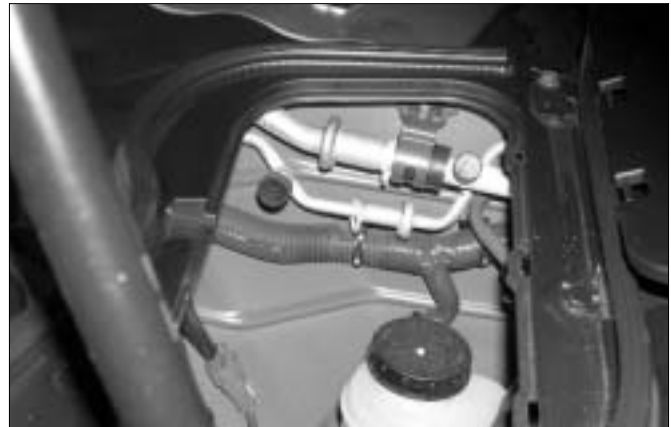
Figure 9. The cover is off and there's the brake fluid reservoir, all right. But both A/C service valves are there too.
